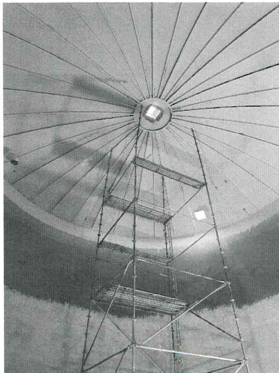
PHOTOGRAPH DESCRIPTION: View of Roof, Angle Stiffeners, Roof Vent, and Roof Hatch.
